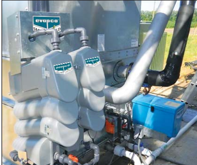
Closed Circuit Cooler Baton Rouge, LA USA
