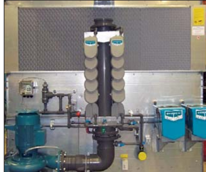
Closed Circuit Cooler Bruges, Belgium
