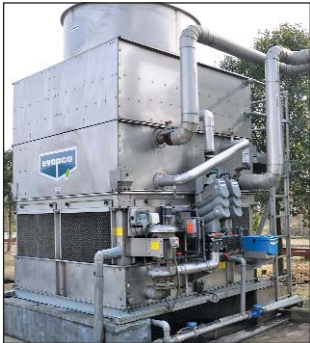
Closed Circuit Cooler Shanghai, China
